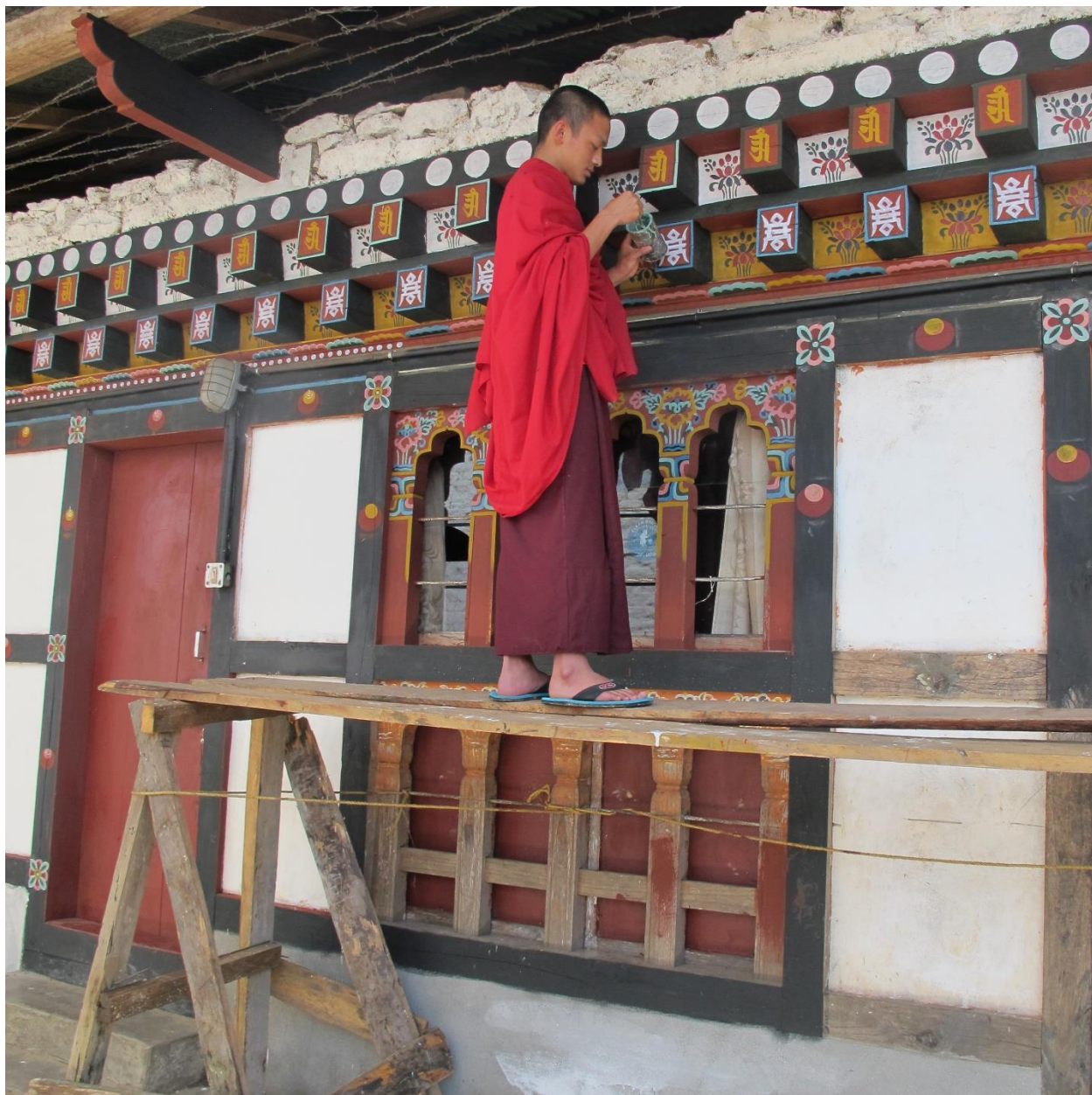
Drametse Lhakang Shakor, Bhutan, during reconstruction (Image: Bhutan Foundation and Division for Conservation of Heritage Sites, Department of Culture/World Monuments Fund)
