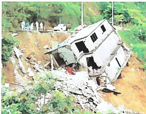
Fig. 3.7. House collapsed. Inappropriate construction practices and construction in unstable land increased the physical vulnerabilities of the region.
