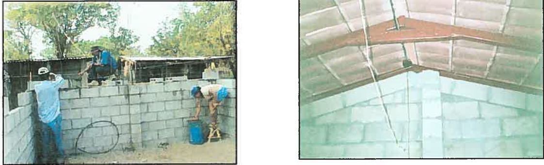
Fig. 3.3 User's labour force was used in construction. Left: the technology chosen for most of the units was labour intensive. Right: detail of the interior of a house. Even though training in construction was provided, many construction defects resulted from the use of unskilled labour.
