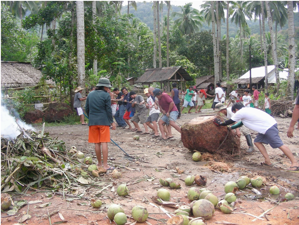
Picture VI.5. Tagbo in Acasia. Clearing of tree stumps to concrete a common space
