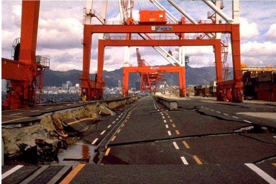
Figure 16: Damages resulting from liquefaction to port infrastructures at the port of Kobe following the January 17 1995 earthquake.
