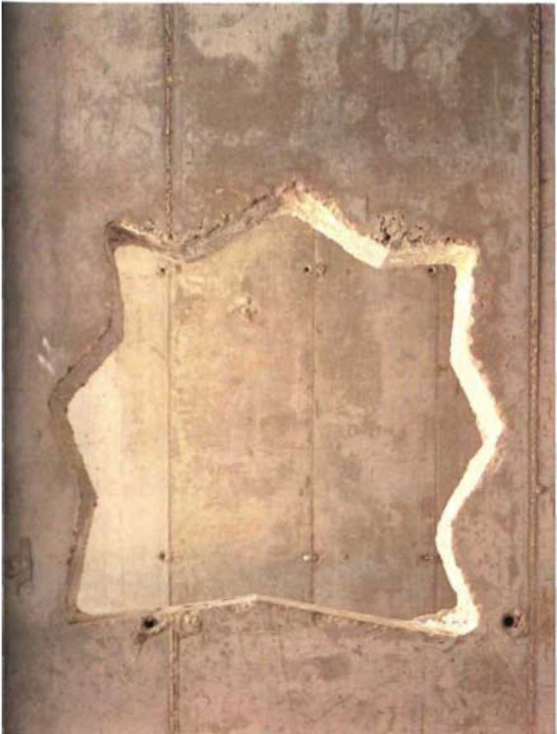
Figure 14 : Star-shaped hole in a wall caused by “worming” in one of the fake ‘Arab’ homes in Chicago 34
