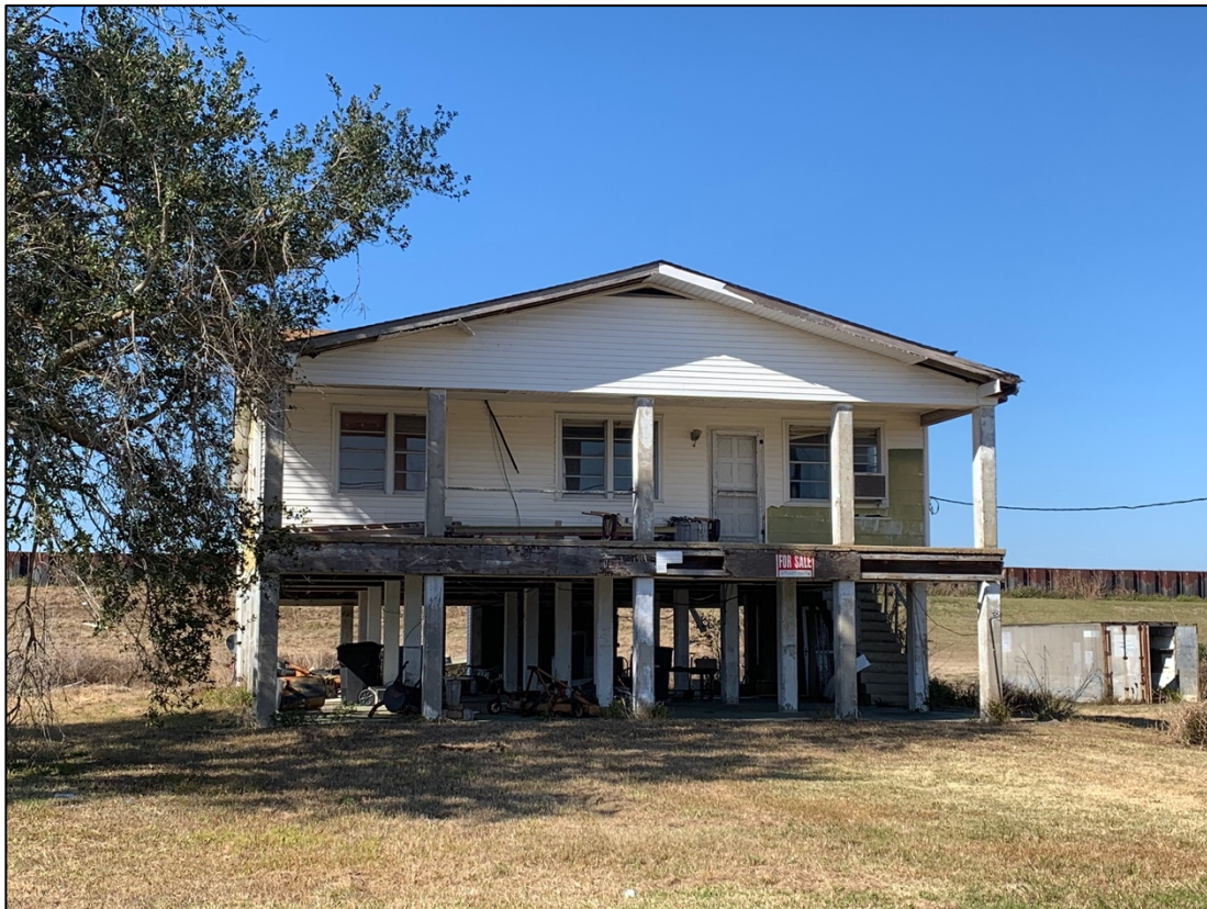
Photo 20. - A stilted home for sale, damaged by Hurricane Ida, Plaquemines Parish
