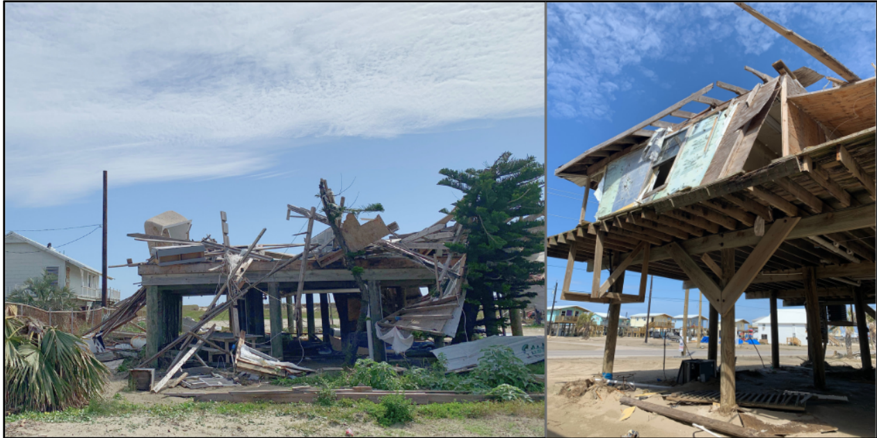
Photo 16. - Houses damaged by Hurricane Ida, Grand Isle
