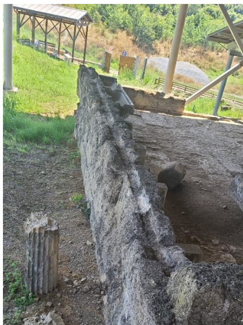
Fig. 16- Conduits in the Northeastern wall of the palaestra , Gymnasium , Amphipolis (Personal Archive)
