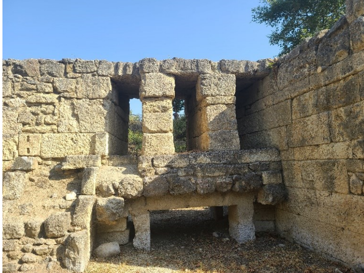
Fig. 55- Classical gate transformed into a large water conduit, Northern fortifications, Amphipolis. (Personal Archive)
