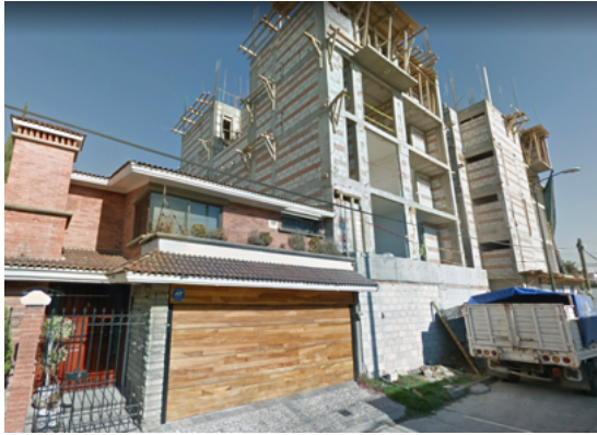
Figure 4: A new apartment block being built next to an older house Source: Google Streetview
