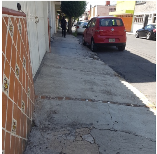
Figure 18: Uneven car ramp
