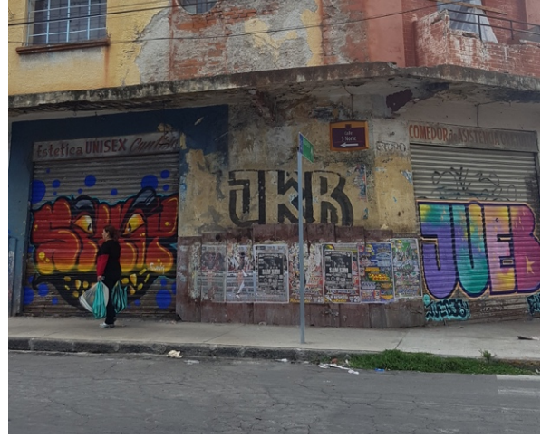
Figure 6: Degradation and vandalism in El Refugio
