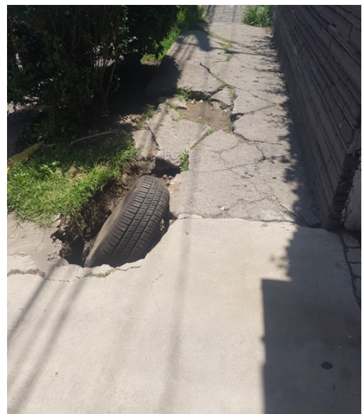
Figure 19: Hole in sidewalk and detritus
