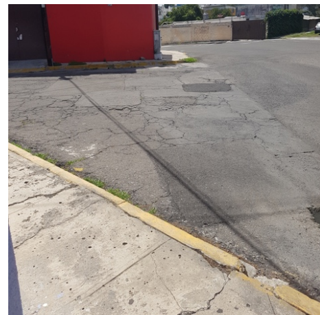
Figure 23: Absence of pedestrian infrastructure at an intersection
