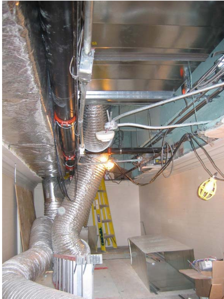
Figure 7- One credit for the design and installation of mechanical and electrical infrastructure in heritage buildings in a way that ensures the sustainability of cultural heritage significance.
