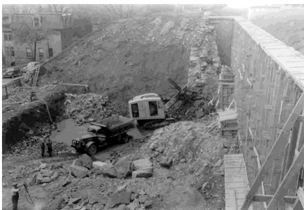
Figure 2.37 McTavish reservoir reconstruction, ca. 1950 With new concrete wall and trace of old stone wall on south side
