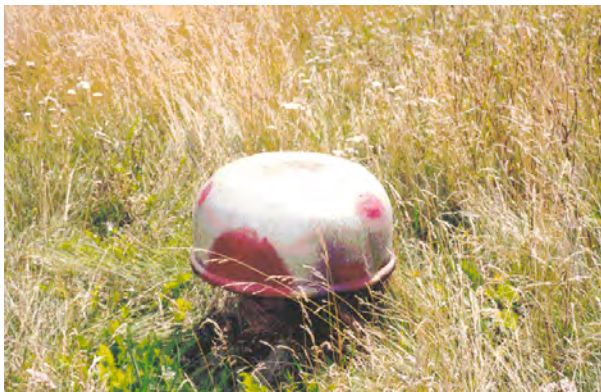
Figure 5.17 Côte-des-Neiges reservoir ventilation outlet/ mushroom Even a discreet signal of the hidden function of the reservoir is camouflaged.
