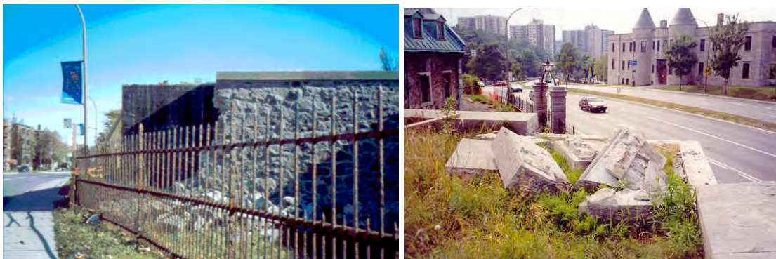
Figure 5.7-8 Côte-des-Neiges reservoir stone wall falling down, 2001
