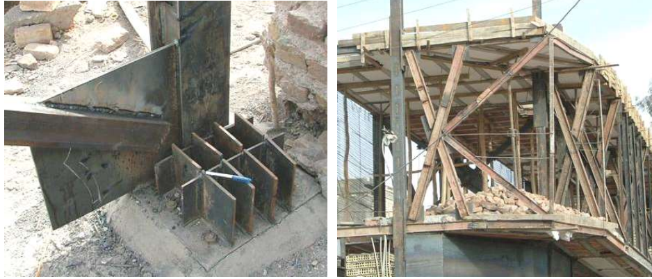
Figure 5.4: Improper use of reinforcement illustrates the lack of safe-construction knowledge – Photos by: M. Gharaati
