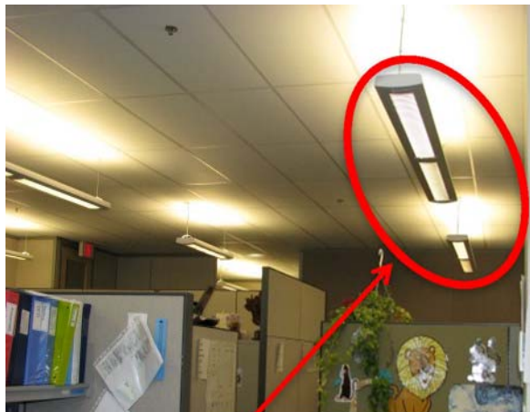
Typical fluorescent lamps in workspaces
