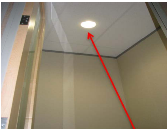
Typical recessed lights (This picture is in phone booths)
