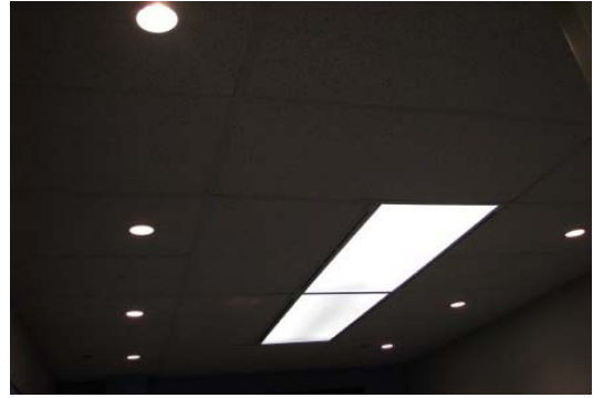
Figure 57. Fluorescent lighting and recessed lights in the GLW
