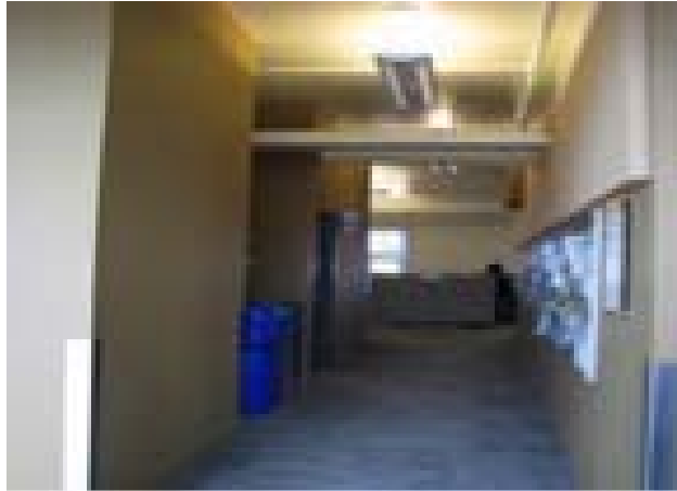
Figure 75. WCB low-voltage fluorescent lighting
