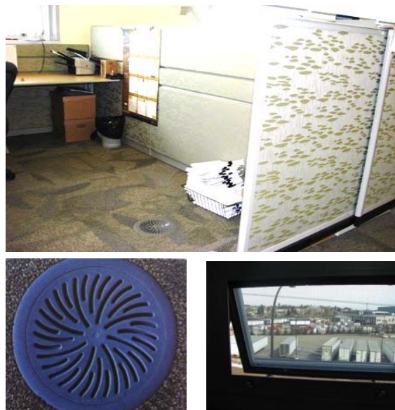
Figure 76. Warm air diffusers and operable windows in the WCB
