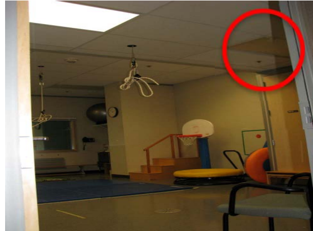
Figure 25. Treatment room with broken light bulb
