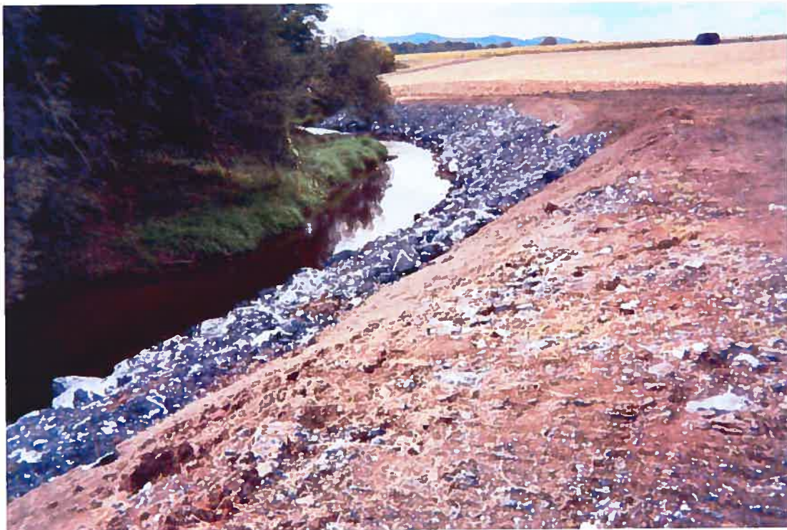
Figure 2: Hard-engineering stabilization technique (rip-rap) used in the Petite Barbué River downstream of the study reach.
