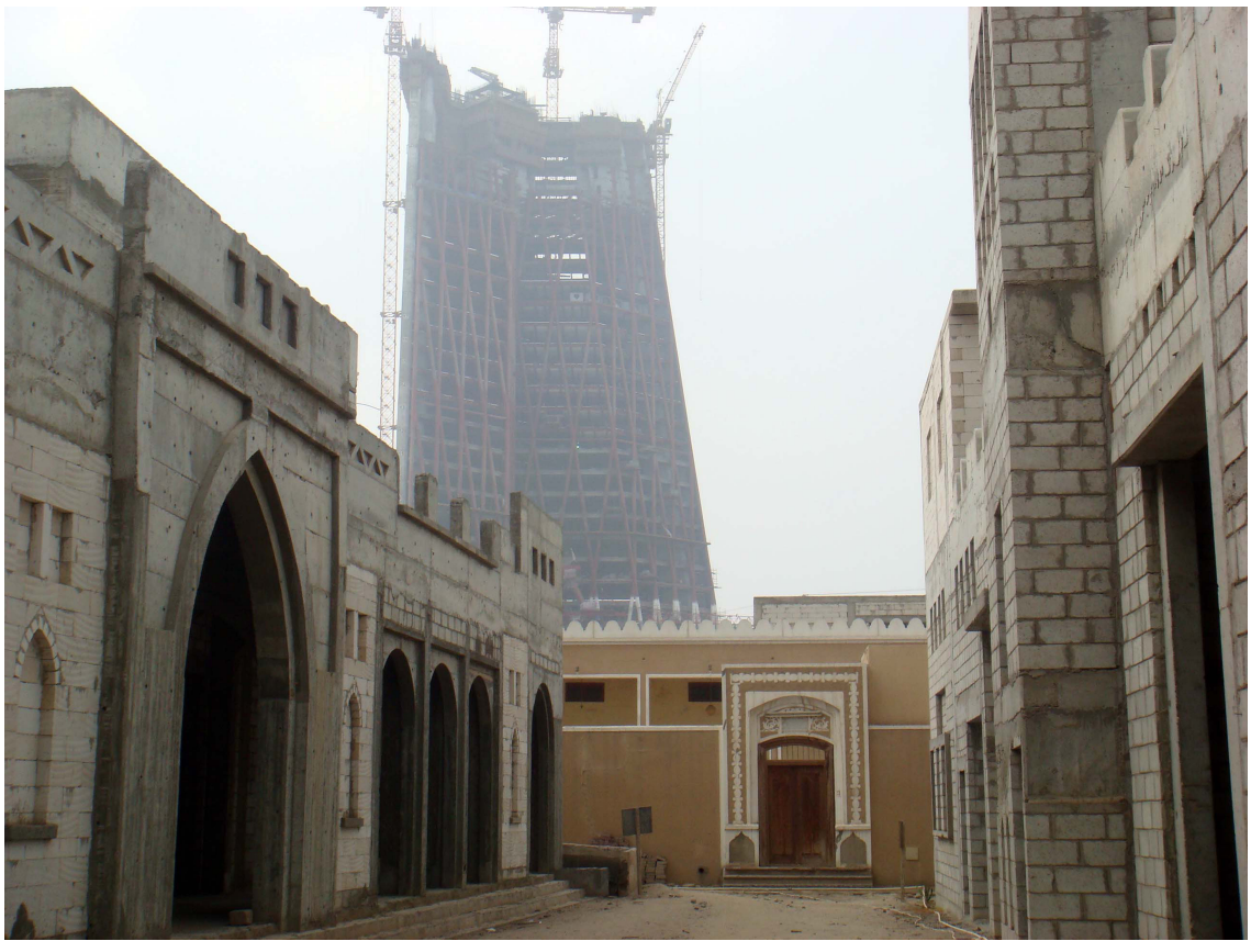
Figure 30: An area between Zones 4 and 5 of the HV. Zone 4 is on the right whereas Zone 5 is on the left. M5 is the mosque in the middle. The CBK, which reached twenty-eight storeys at the time, is in the background (source: researcher, 2011-01-30).
