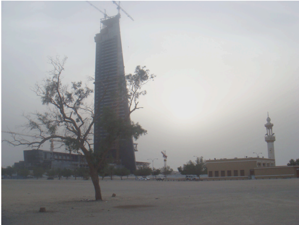
Figure 41: Relationship between the CBK and Said Abdullah Mosawi mosque. The KIA will be constructed across the street from that mosque (source: researcher, 2012-05-28).
