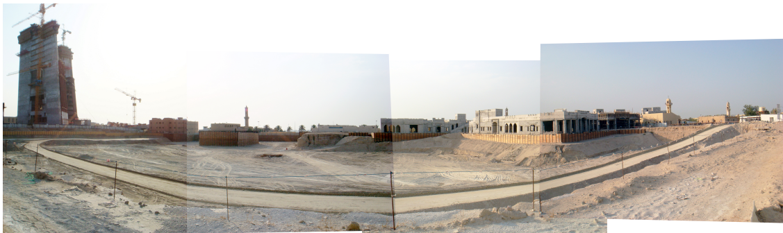
Figure 25: Panoramic view inside the HV. The CBK is on the left. Zone 4 of the HV is under construction (source: researcher, 2010-08-08).
