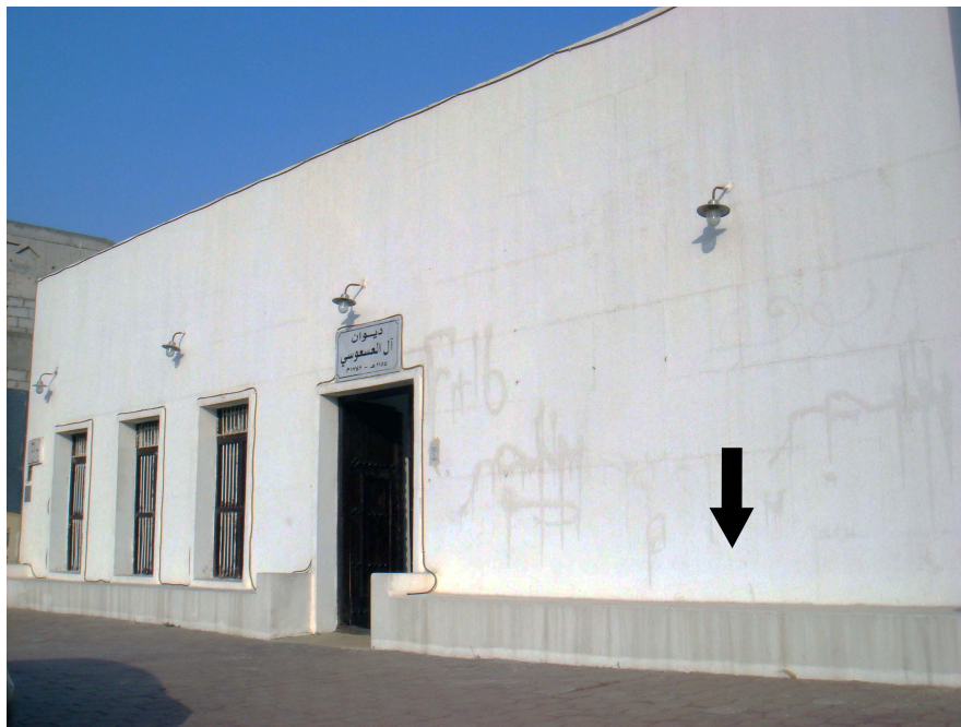
Figure 9: Dacha attached to the façade (facing the harbor) of Al-As'oussi Diwan , which is a heritage building in Kuwait City (source: researcher, 2011-01-18).
