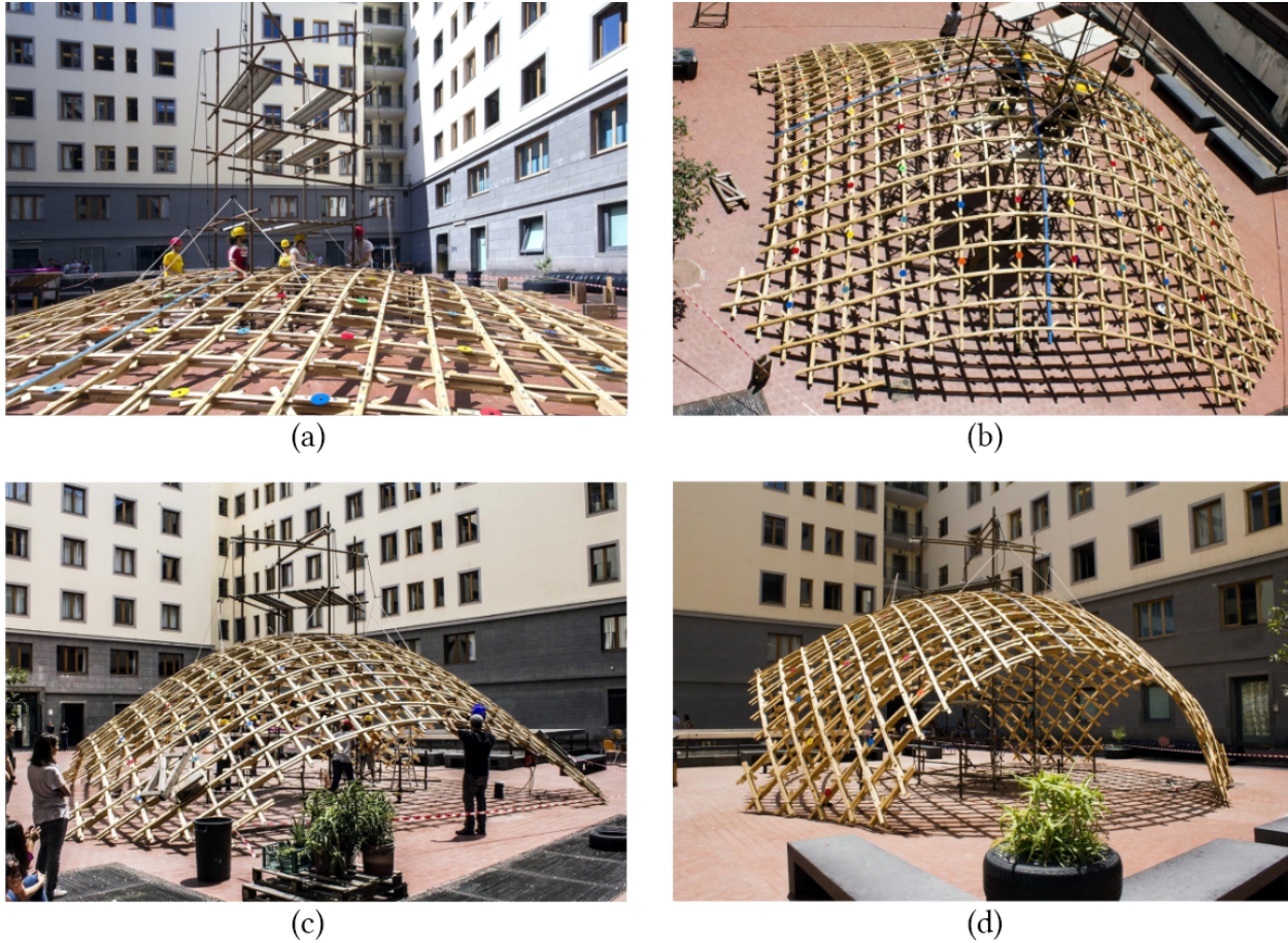
Fig. 1.4. Deployment of the Toledo gridshell 2.0. The gridshell is first assembled on a flat surface (a), before being deployed (b,c). The fully deployed gridshell (d) stands on its own (scaffolding was later removed). This figure is taken directly from [D’Amico et al., 2015].
