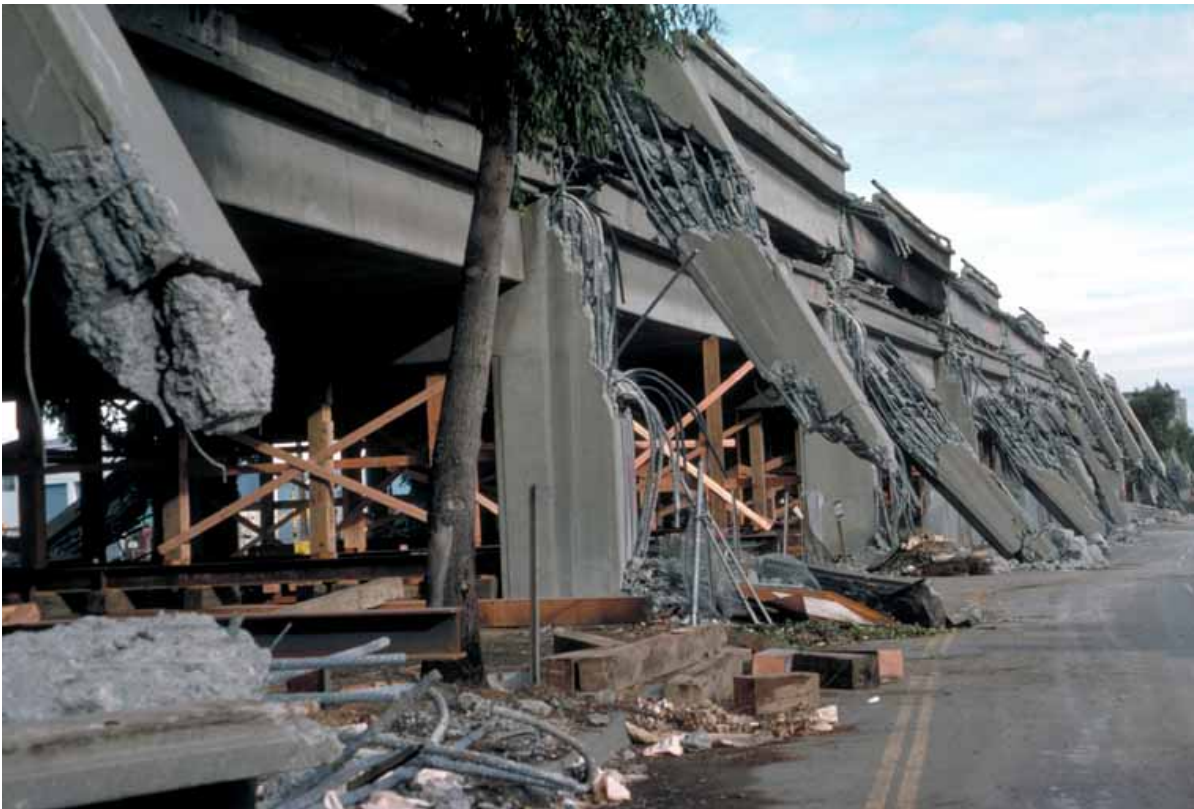
Figure 66. Collapsed Cypress Street Viaduct in Oakland, California after the 1989 Loma Prieta Earthquake, a grim omen of what could happen in Seattle. Created by H.G. Wilshire, U.S. Geological Survey, 1989. From Wikimedia Commons. https://commons.wikimedia.org/wiki/File:022srUSGSCyprusVia.jpg
