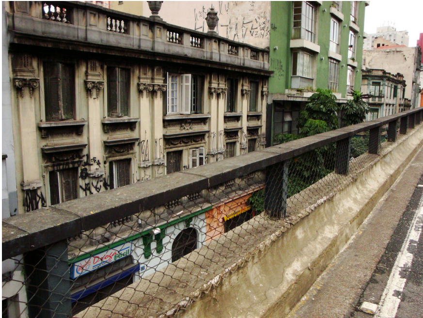
Figure 77. Photo showing proximity of elevated freeway to deteriorating facades of historic residences, showing both decline of neighborhood and illustrating the issue of noise pollution with traffic so close to bedrooms. Photo taken by Milton Jung, 4 April 2010. From Flickr. https://www.flickr.com/photos/cbnsf/4516297606
