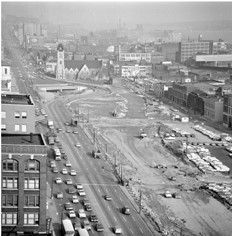
Figure 24. Demolition of a historical neighborhood in Detroit as part of the mid-century slum-clearance campaigns. Photo from Walter P. Reuther Library, accessed on Curbed Detroit. https://wdet.org/media/daguerre/2015/10/18/b6533dbcle32eb51abd.jpeg
