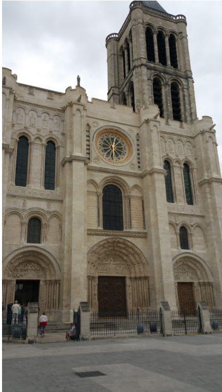
Figure 1. Abbey Church of Saint-Denis showing missing tower lost due to poor structural reinforcement. Photo by Brooks C. Piper, September, 2015.
