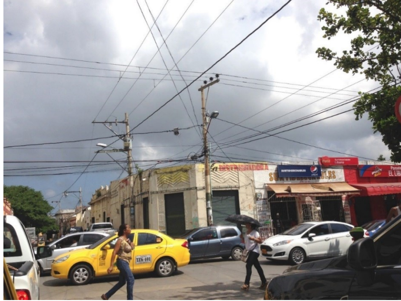
Figure 4 - Light pole and distribution transformer.
