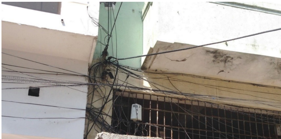
Figure 9 – Electricity distribution grid in subnormal Barranquilla. Detail.
