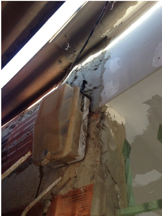
Figure 17 – Electricity meter. Detail.
