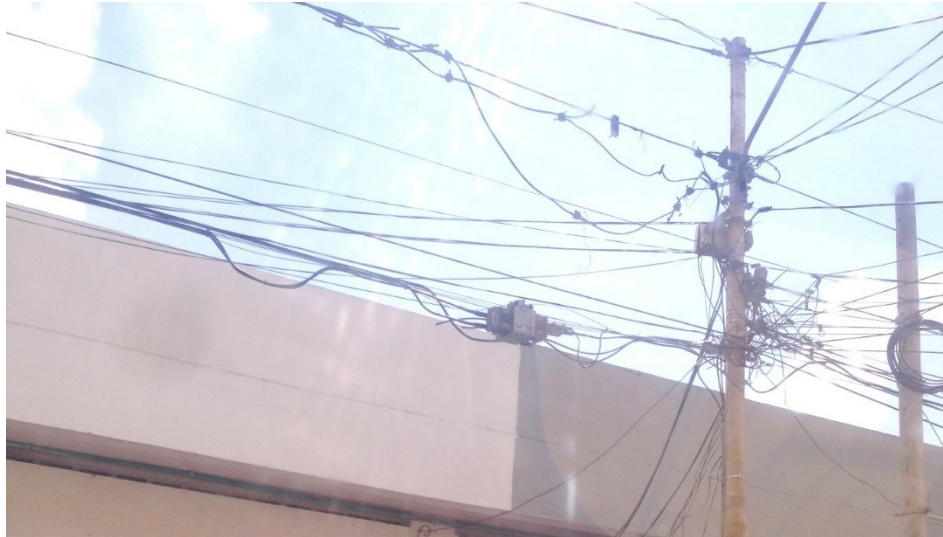
Figure 8 – Electricity distribution grid in subnormal Barranquilla. Detail.
