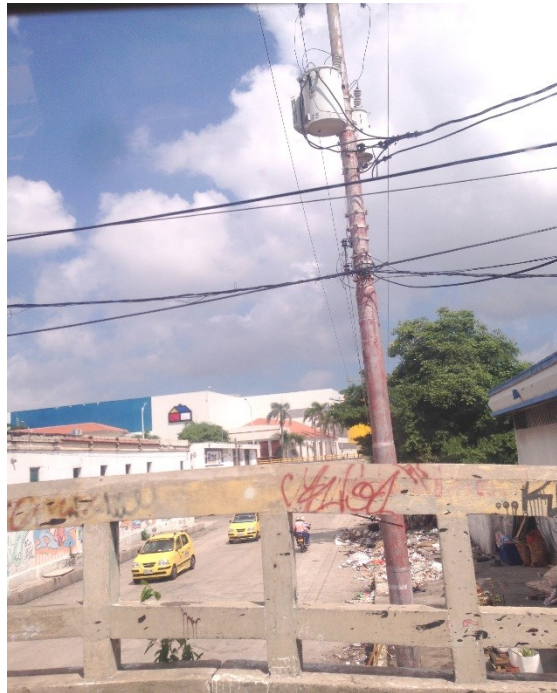
Figure 6 – Distribution transformer in the city center.
