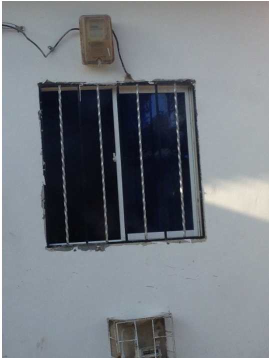
Figure 16 – Electricity meter. Detail.
